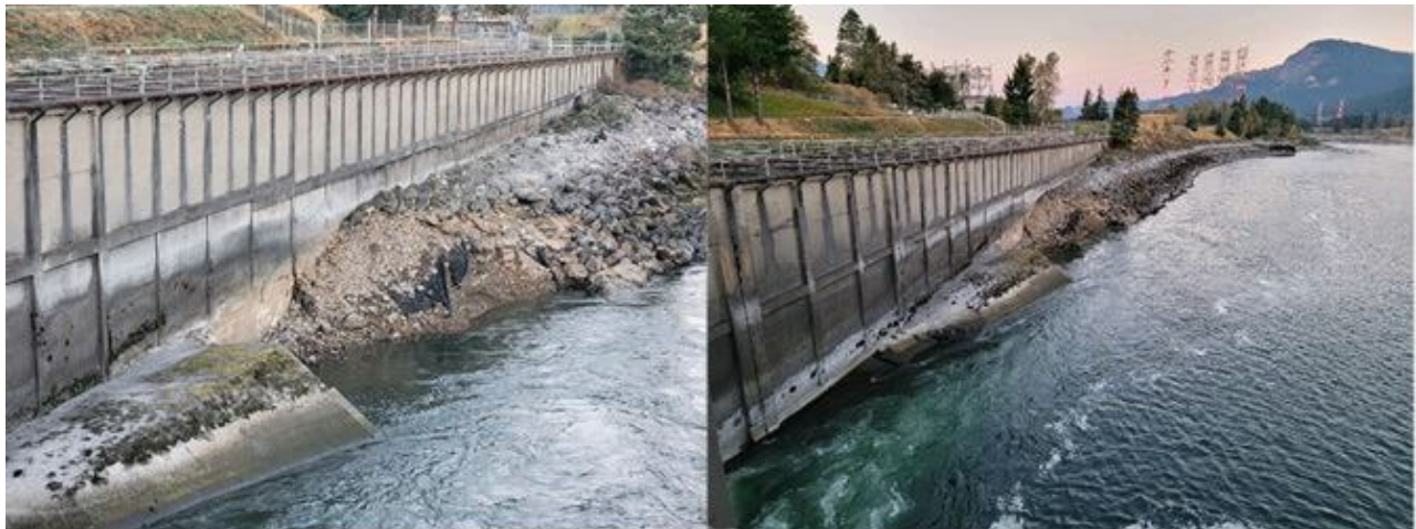
Photo 1: Left frame, close photo of damage to the B-Branch Fish Ladder apron. Right frame, overall photo of the damage. Photo obtained from MOC 22BON089.
